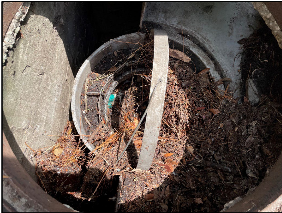
Photograph 9: Accumulation of sediment and debris in inlet basket at the intersection of Killarney Drive and Salisbury Boulevard
