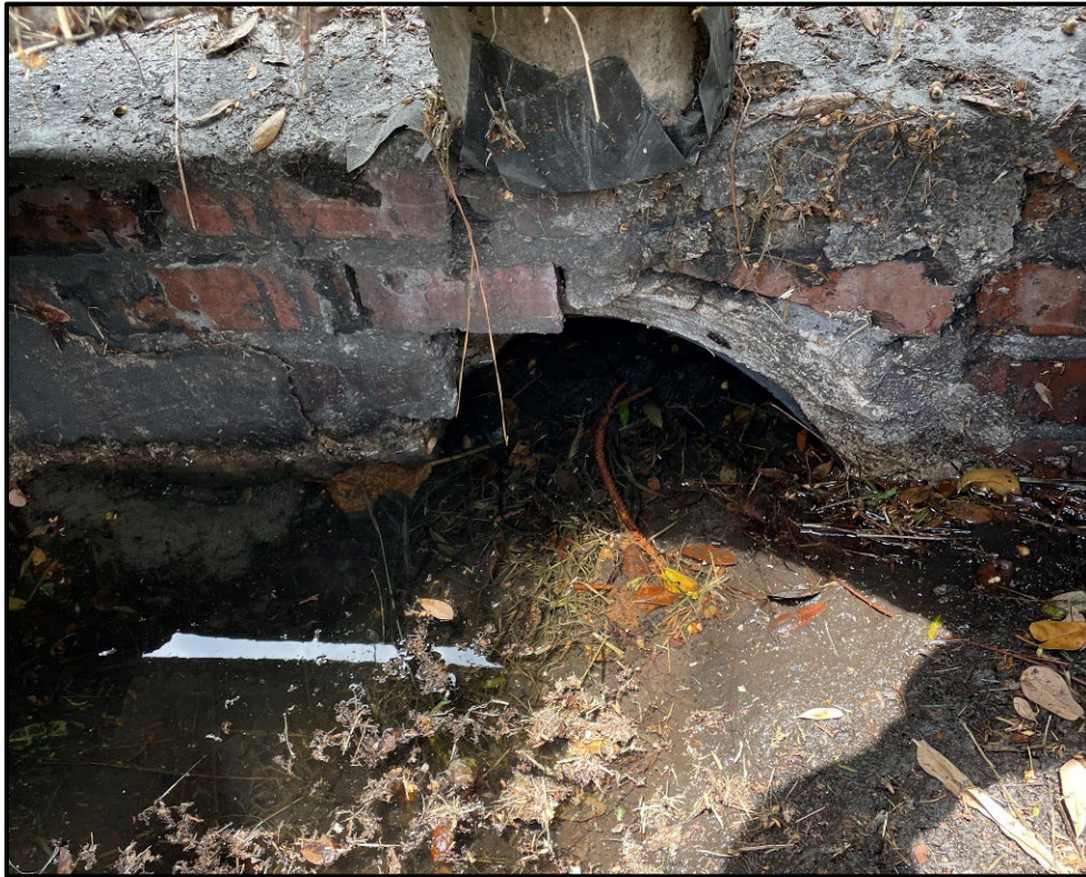
Photograph 6: Upstream side of reported collapsed 12-inch steel pipe at the east end of Euston Road
