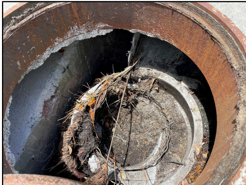
Photograph 3: Accumulation of sediment and debris in inlet basket at the intersection of Pelham Road and Euston Road
