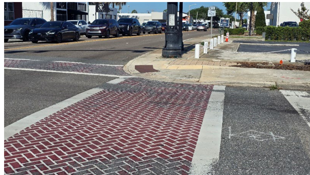
Crosswalks, tactile pavement and curb in need of repair at northeast corner at the intersection of Pennsylvania Avenue and SR 426
