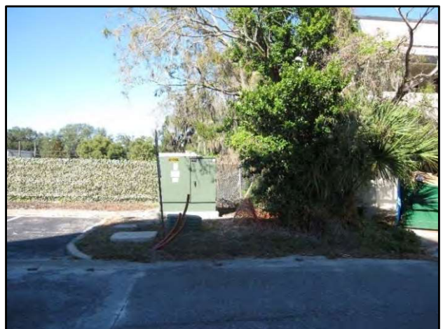
The subject's approximately 19' frontage on Swoope Ave is obstructed by an electric transformer recently installed in the right-of-way.
