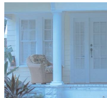
Replacement column not consistent with building style
