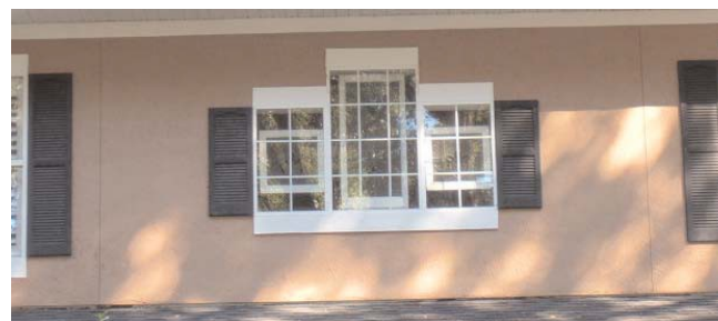
Inappropriate Window Type
