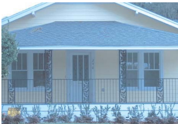
Porch supports not consistent with style
