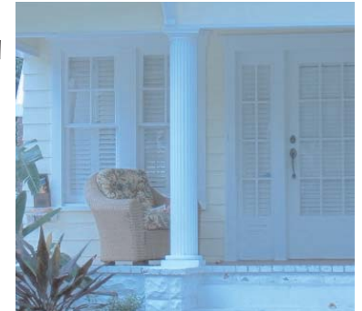
Replacement column not consistent with building style
