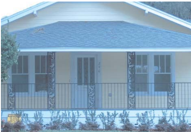
Porch supports not consistent with style
