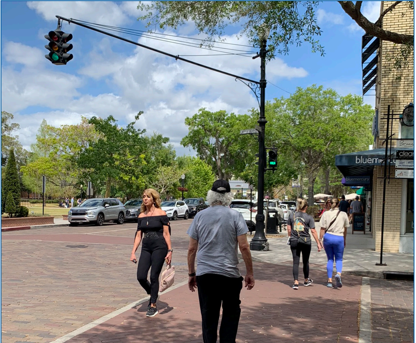
Figure 3 - Legacy traffic signal equipment along Park Avenue
