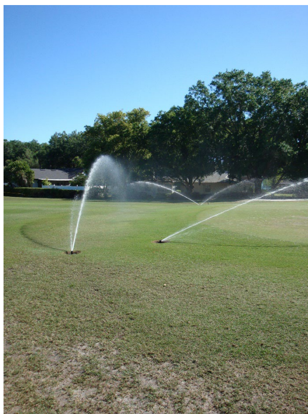
Poor green block sprinkler spacing & coverage
