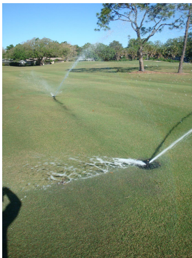
Poor block system fairway & tee sprinkler spacing & coverage
