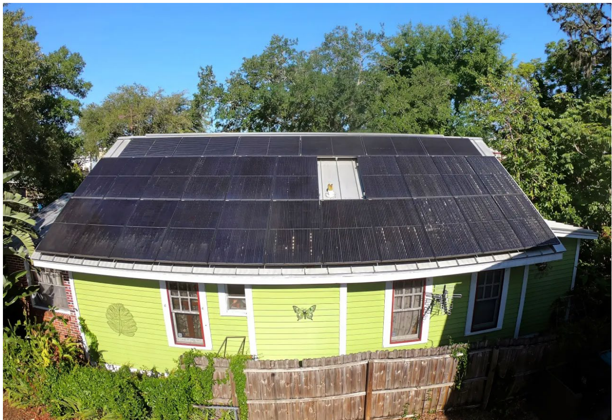
Patty Sheehan, an Orlando city council member, installed solar panels on her home about five years ago. They reduce her power bill to nearly nothing. (Joe Burbank/Orlando Sentinel)
