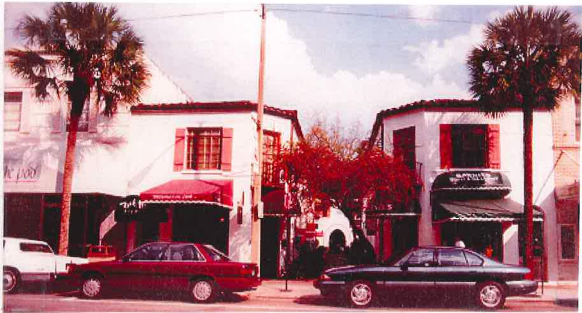
Inappropriate Use of Awning: Awning Placed over Another
