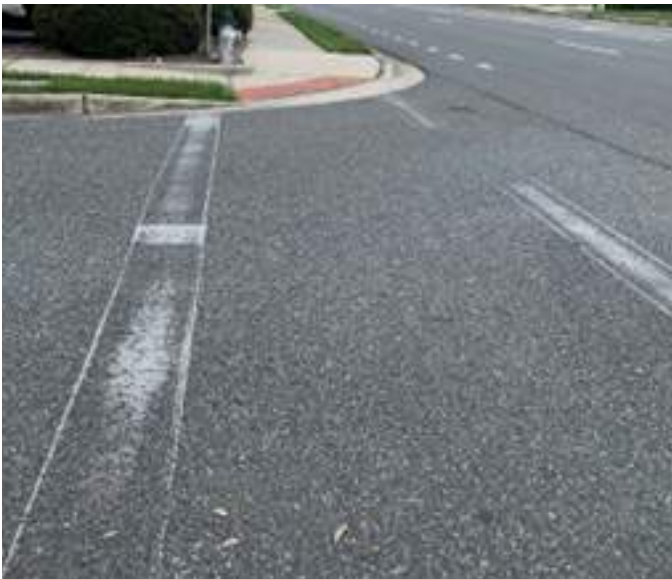
Deteriorated cross-walk markings.
