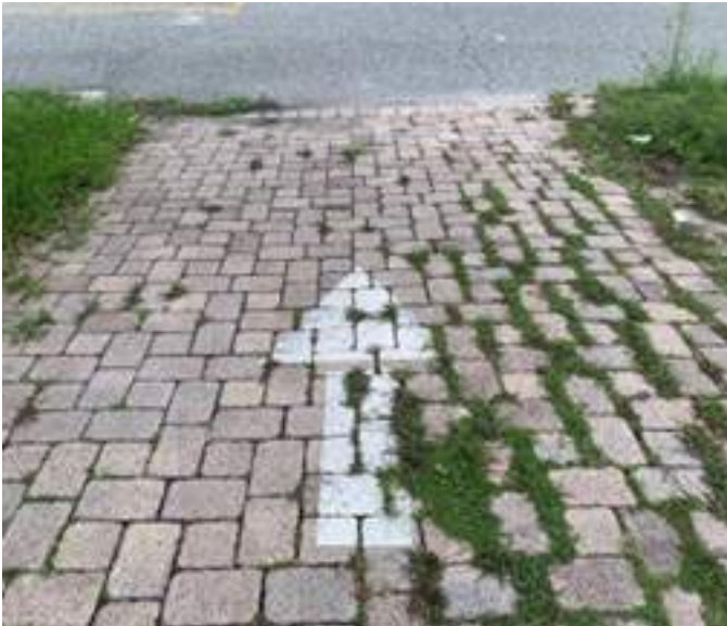
Deteriorated brick driveway.
