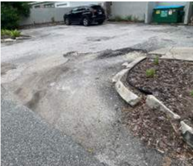
Deteriorated parking lot entry apron and curb.
