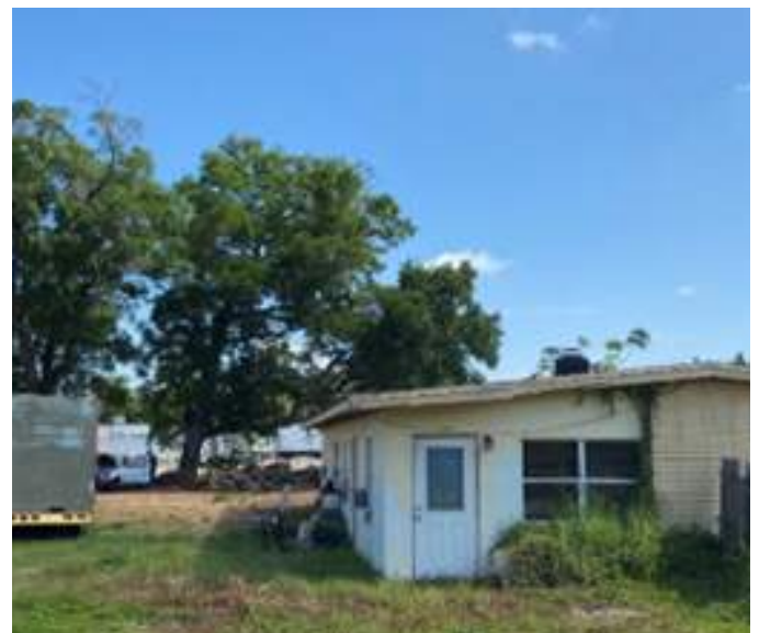
Deteriorated building and site improvements.
