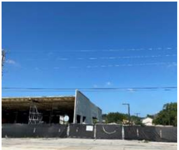
Examples of deterioration of site improvements, electric switch boxes, public parking, private development and curb cuts/driveways
