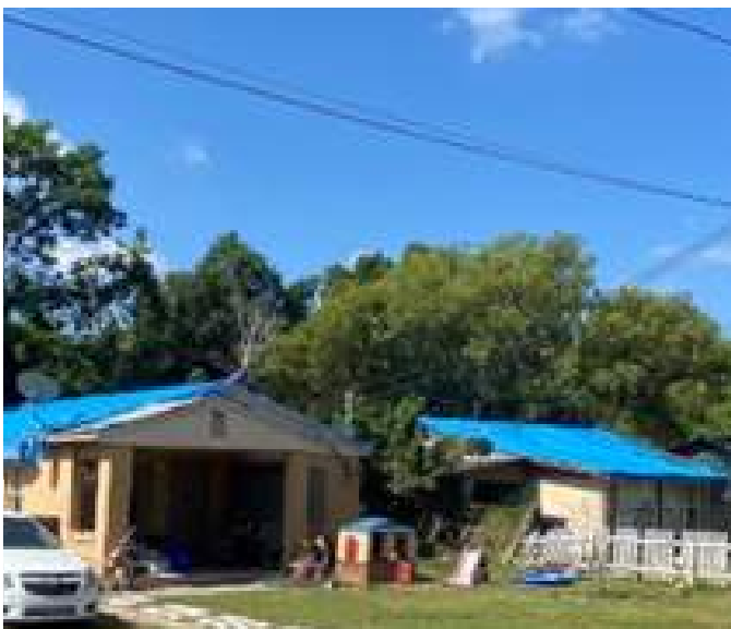
Deteriorated building and site improvements.
