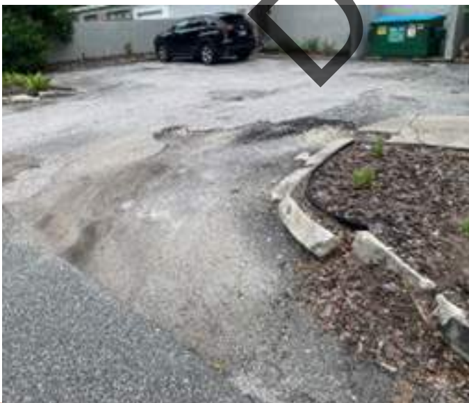
Deteriorated parking lot entry apron and curb.
