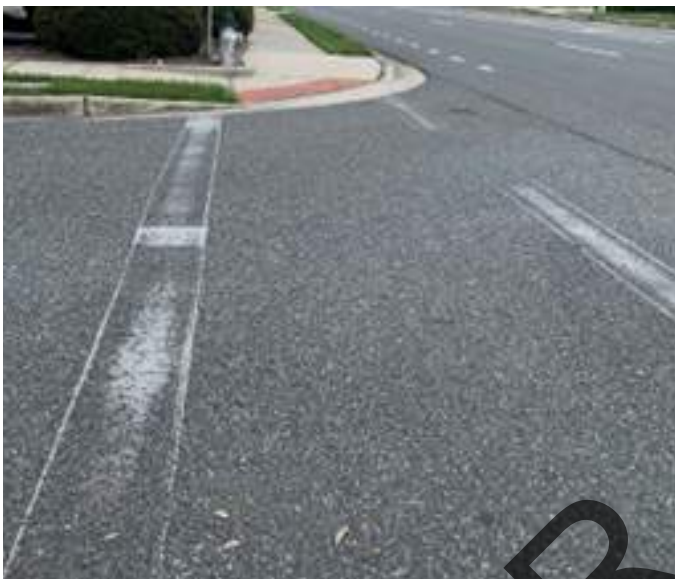
Deteriorated cross-walk markings.
