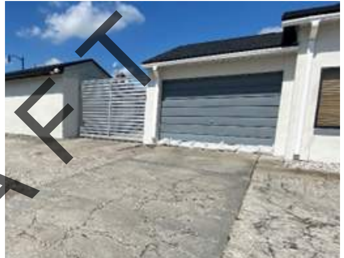
Deteriorated signage and parking improvements.
