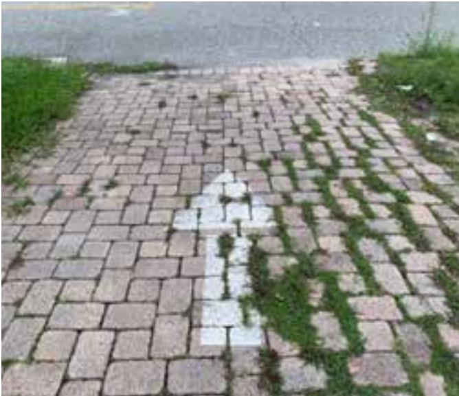
Deteriorated brick driveway.
