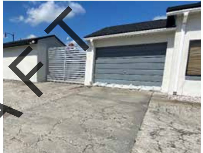
Deteriorated signage and parking improvements.
