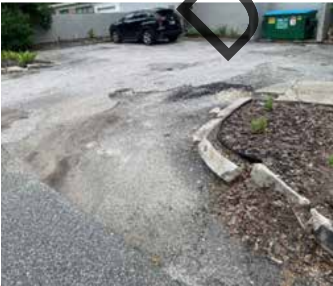
Deteriorated parking lot entry apron and curb.
