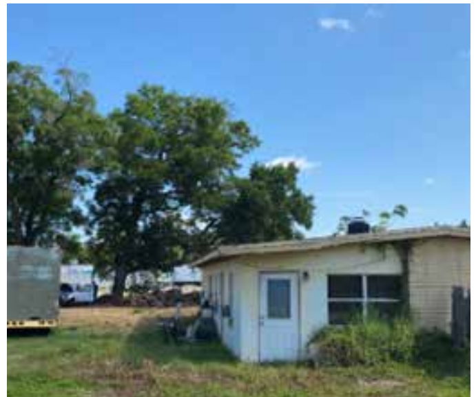
Deteriorated building and site improvements.
