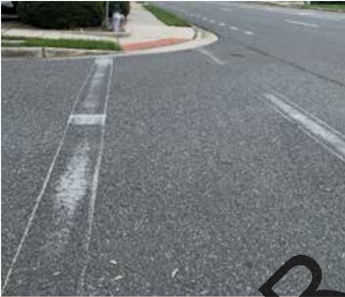
Deteriorated cross-walk markings.
