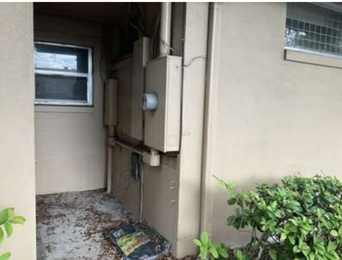
Typical view of metered area
