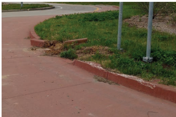
Figure 7. Curb damage on center island of a roundabout. (Photo source: MRIGlobal.)
