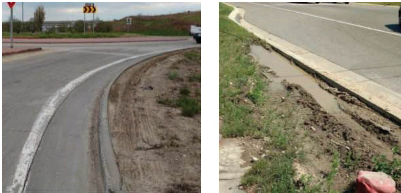
Figure 6. Rutting resulting from truck encroachment at a roundabout approach and rutting resulting from truck encroachment at a loon. (Photo source: MRIGlobal.)
