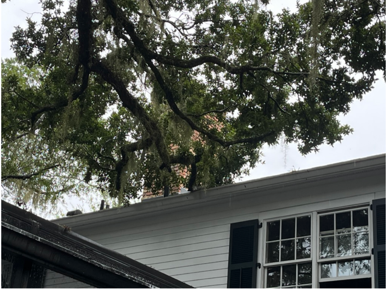
Tree resting on the roof of the house resulting in water retention and added stress to the roof structure, and damage to the existing gutter system.
