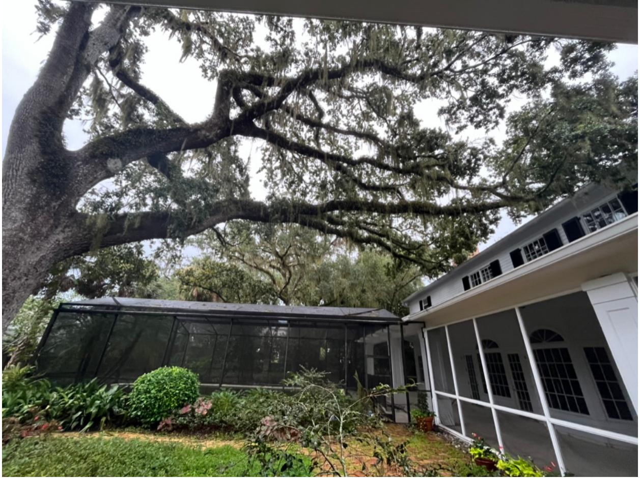
Tree resting on the roof of the house in several locations.
