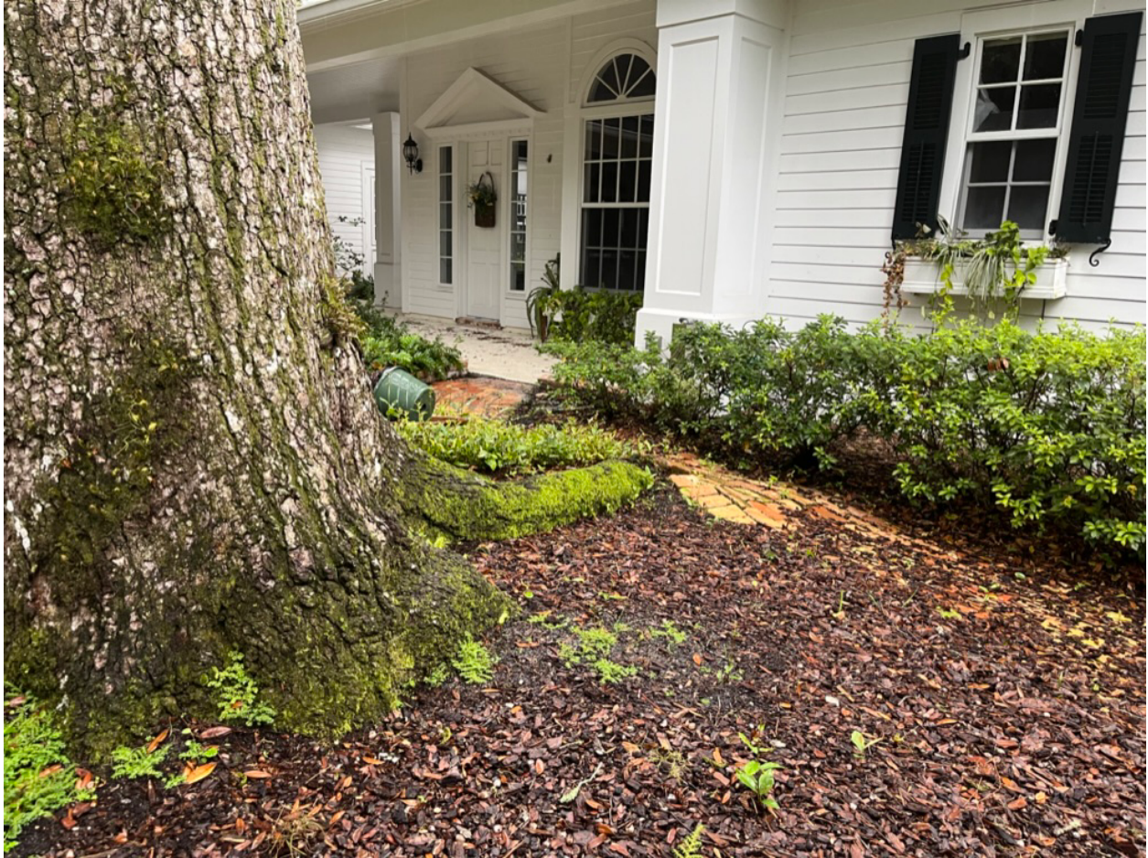
Note the root system growing towards the guest house (currently visible distended from the ground roughly 3' from the existing foundation).
