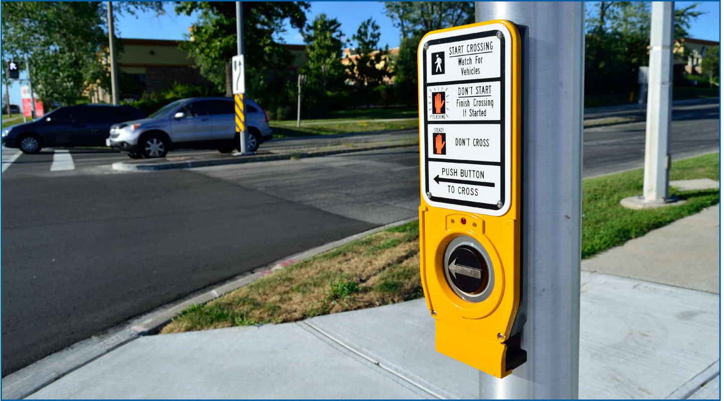
Figure 10 - Accessible Pedestrian Signal (APS) push buttons. ( https://commons.wikimedia.org/wiki/File:PedestrianSignalPushButton.jpg )
